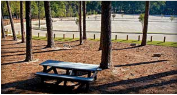
Figure 3. A large PICP parking lot manages an overall site slope of 12% using terraced areas.
